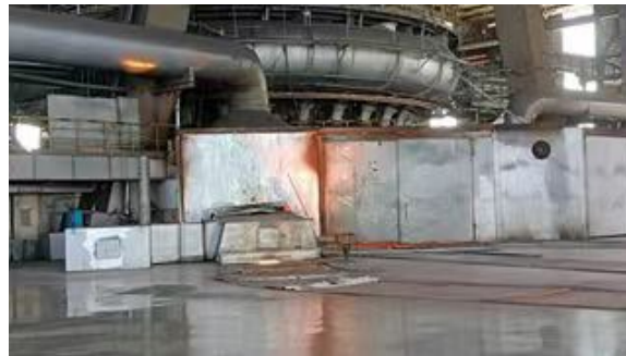
Fig.12. The Dust removal effect on production site
